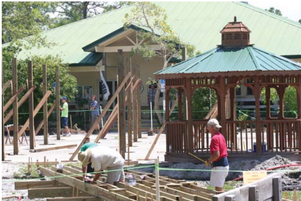
Top to Bottom: ECHO Tropical Fruit Nursery Sign; Interns Kimberly Duncan, Laura Catherine Conville, Brandon Lingbeek and Asst. Farm Manager Joel Wildasin harvest bamboo for railings for the boardwalk; Boardwalk, shade cloth supports and gazebo in progress.
